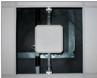
Files are automatically tracked as they arrive by sensors in the ceiling.
